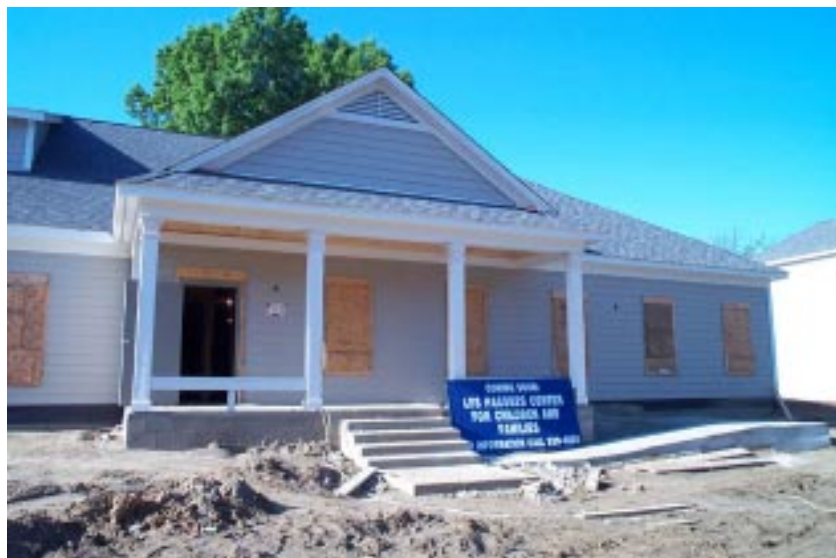
MIFA is working with a consultant to develop an evaluation plan for its Les Passees Center for Children and Families, its new state-of-the-art child enrichment center (seen here under construction).
